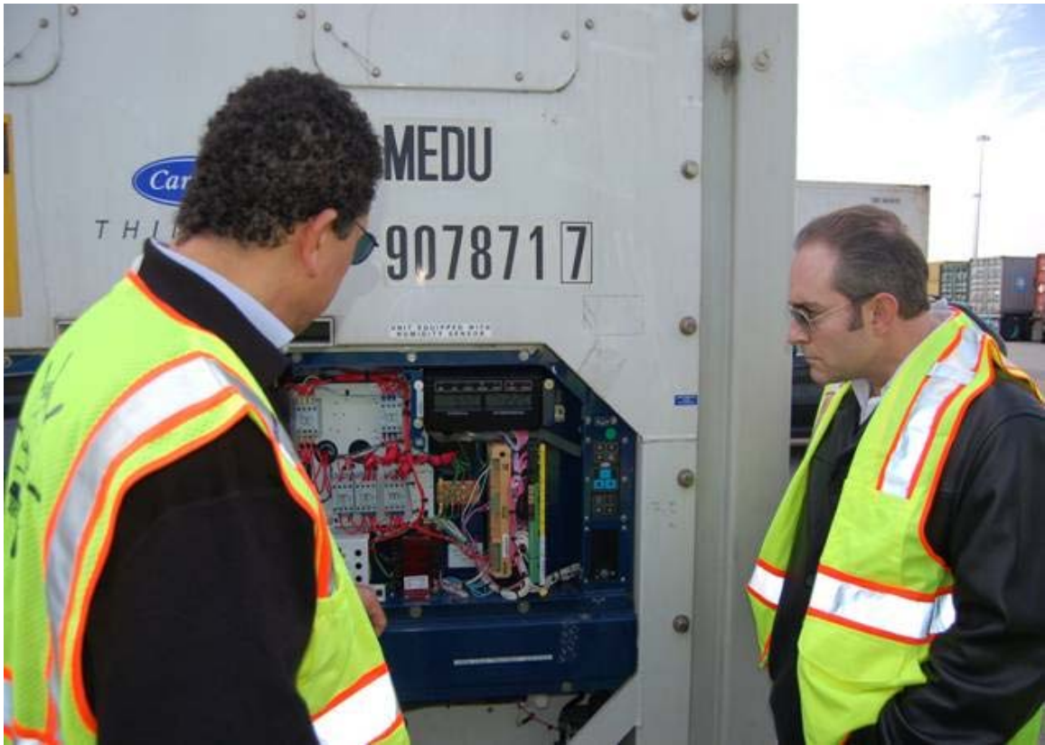
Mostafa Shawki from Mediterranean Shipping Company and Neil Ross from MGM take a glimpse of the inner workings of the reefer's control module.
